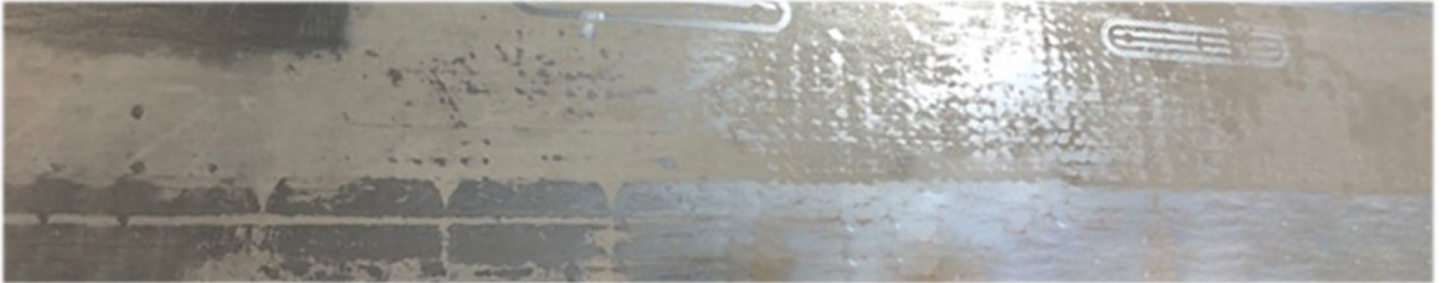
-Image of oxidation on a galvanized subpanel.
