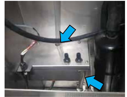
Step 13: After removing the old condensate evaporator assembly slide new unit in place. Connect the two condensate hoses.
