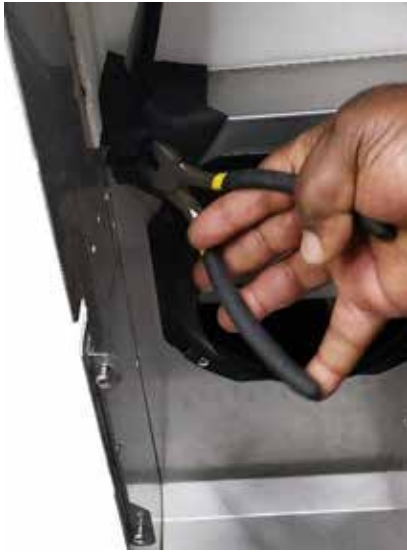
Step 11: The old condensate evaporator assembly can now be removed. Cut cable ties. Cut the cable.
