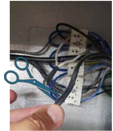
Step 7: Cut the old wire and use to assist in pulling new wire into place
